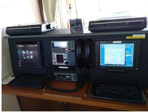
Figure 7: Radio communications console
