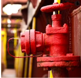
Figure 32: Fire hydrant, on deck.
