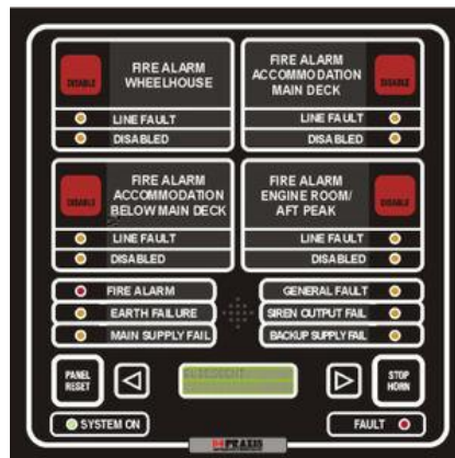
Figure 35: Fire alarm panel.
